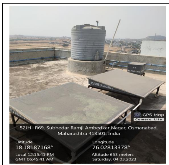
Solar Distillation Plant
