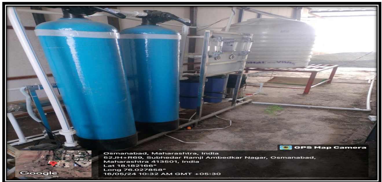
Water RO Plant
